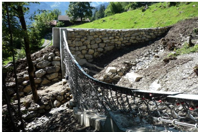
Figure 15. Debris flow barrier in Isenfluh, Switzerland over a population center. The outer bank channel was reinforced with a rock wall
