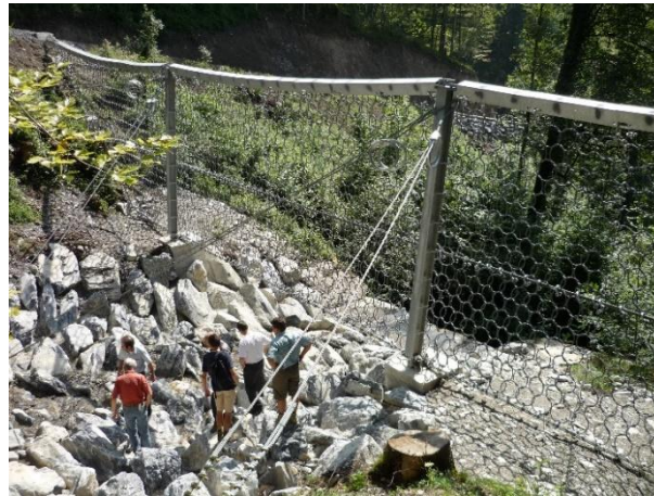
Figure 2. Barrier against debris flow, type UX with posts for the application of wider channels. Trachtbach, Switzerland. Along the riverbed, anti-scour protections (breakwaters and poor concrete) were also placed.
