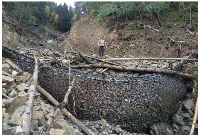
Figure 17. Two of the eleven stepped barriers located in Portainé, current state after 12 years of continuous work, Portainé Spain
