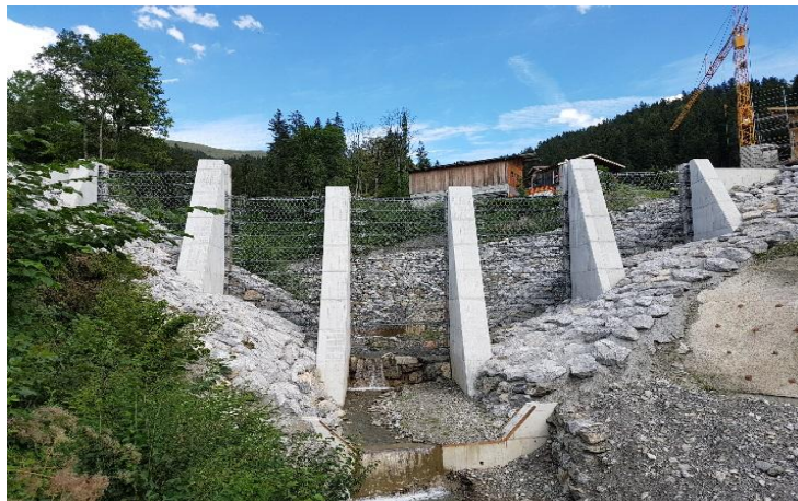
Figure 25. Another special solution acting as a barrier against the flow of debris in Sitäbach, Switzerland consisting of concrete piles combined with ring nets
