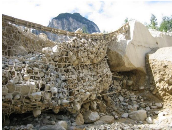
Figure 7. Washed side anchorage, barrier in the Illgraben canal, Switzerland. Partial lateral anchoring in loose material and old disused concrete breakwater
