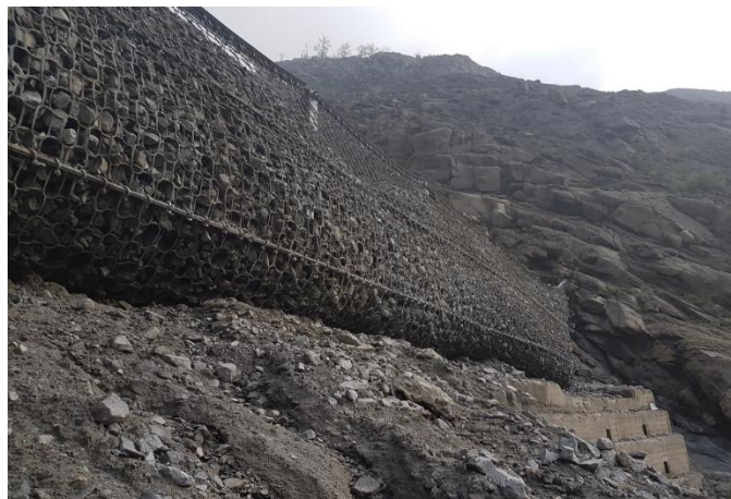
Figure 18. UX barrier after 2017 events in Chosica, Peru
